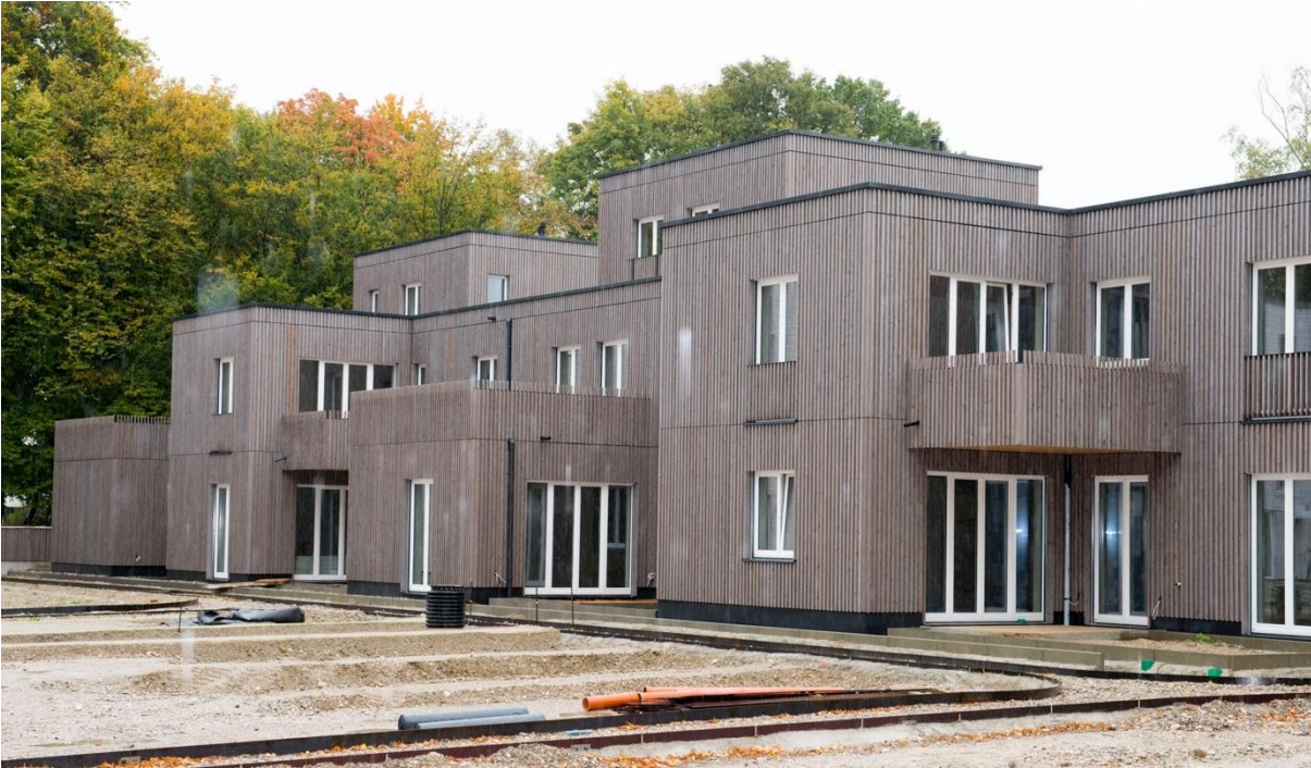
Figure 3.22 Modern timber frame building (2019) in the newly developed residential area “Prinz-Eugen-Park” in Munich (Photo: Ralf Rosin, TUM)
