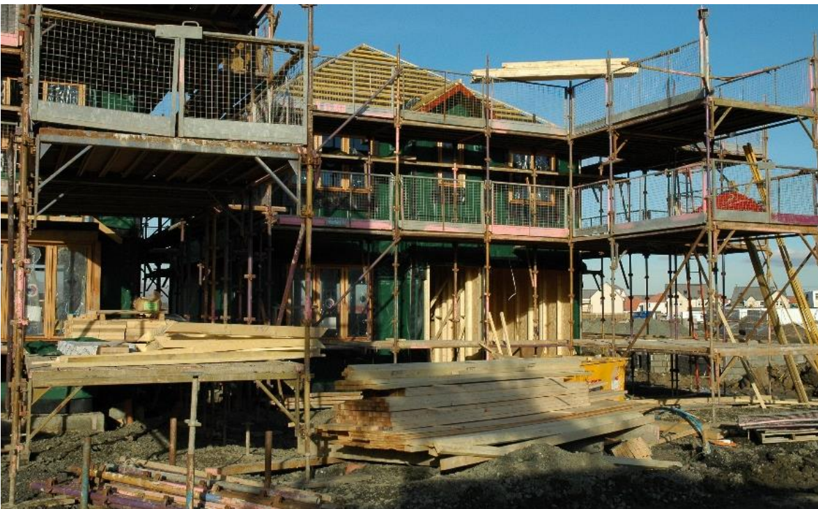
Figure 3.17 Modern timber house construction in Scotland, year 2005, light-frame and prefabricated panels (Photo: D. Ridley-Ellis)
