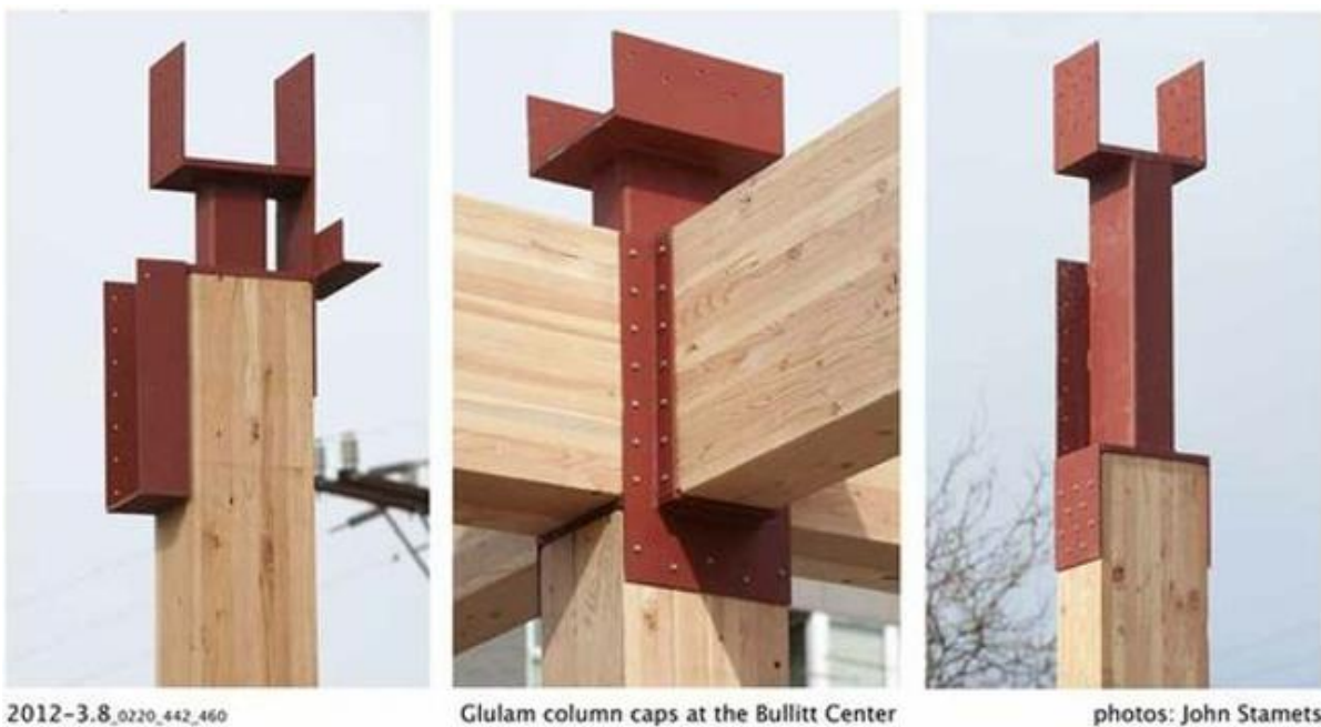
Figure 3.30 Glulam beams with metal connections, Bullitt Center (Courtesy of Bullitt Center, photos by John Stamets).
