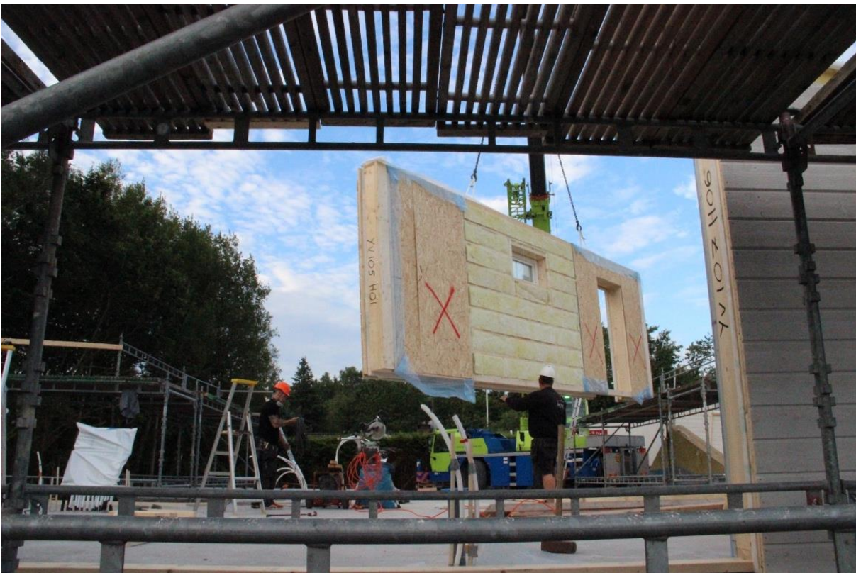
Figure 3.7 Lifting of large prefabricated wall element in Sweden (Courtesy of Derome AB)
