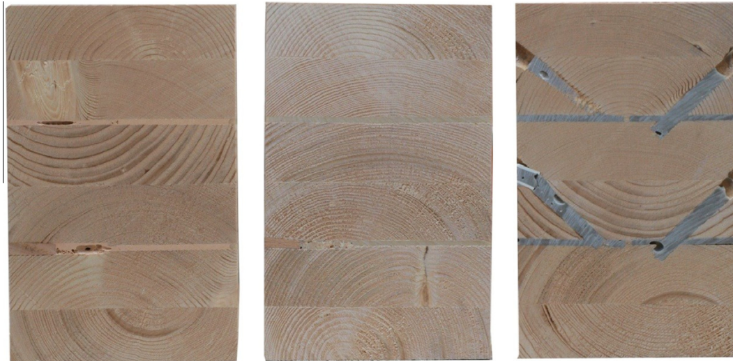
Fig. 16. Result of different repair methods (pouring and injection) for different adhesives, CSA Resin n'H Lungern (left), Purbond RE 3040, RE 3064 (middle), Jowat 692.30 (right), [13].
